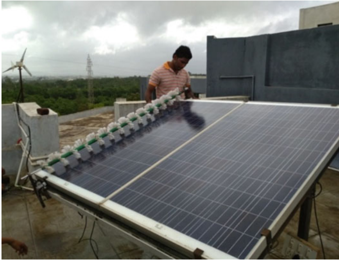
Fig. 7 Test setup of solar PV
